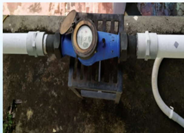
Installed water flow meters in the process line of seafood industry
